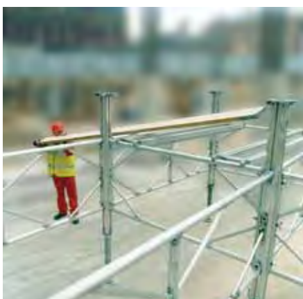
7. Place intermediate transoms and scaffold boards in position for fixing of aluminium beams.
